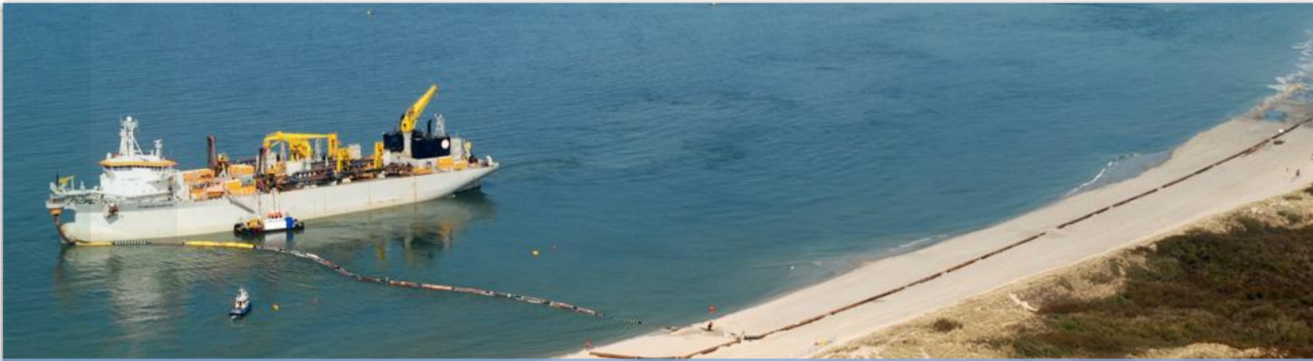
TSHD Charles Darwin dredging for the Dutch Coastal Protection Program (The Netherlands)
